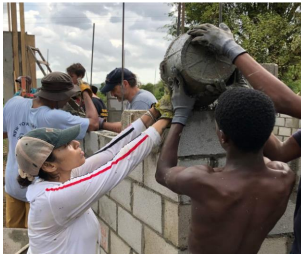
Loose or “soupy” concrete being poured by buckets into the blocks to stabilize the rebar
