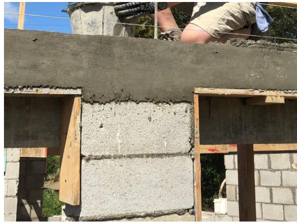
Horizontal column made of thick concrete on top of cinder block with vertical rebar
